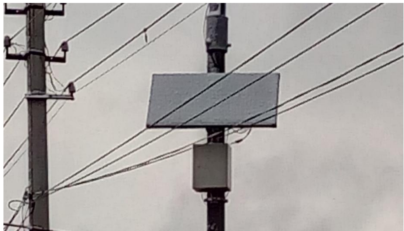
Fig. 2 – Surface contamination of the PV
