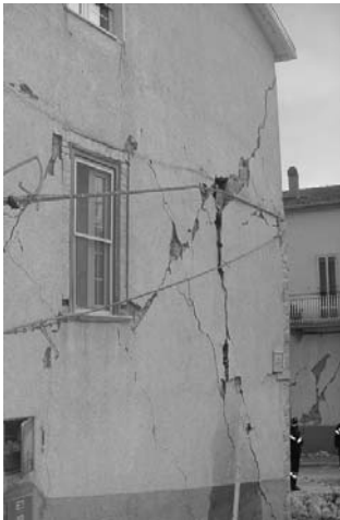
Fig. 16.5. An example of unusable building
