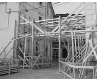
Fig. 16.19. Wooden protected passage (Molise 2002)
