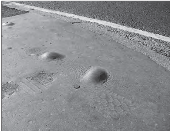
Fig. 1. Asphalt blisters on pavements of London.
